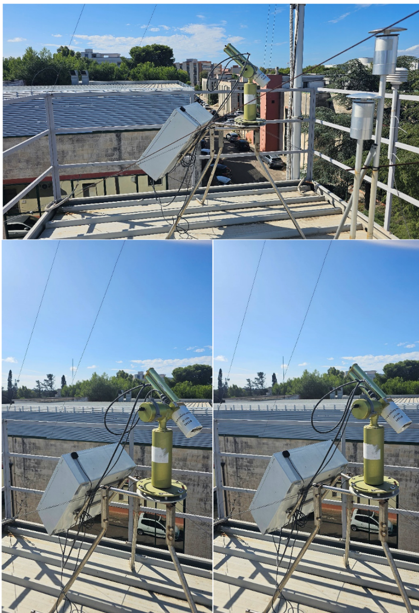
Figure 15: View of the Sun/sky/lunar photometer CIMEL CE318-T located on rooftop of CNR-ISAC Lecce building
