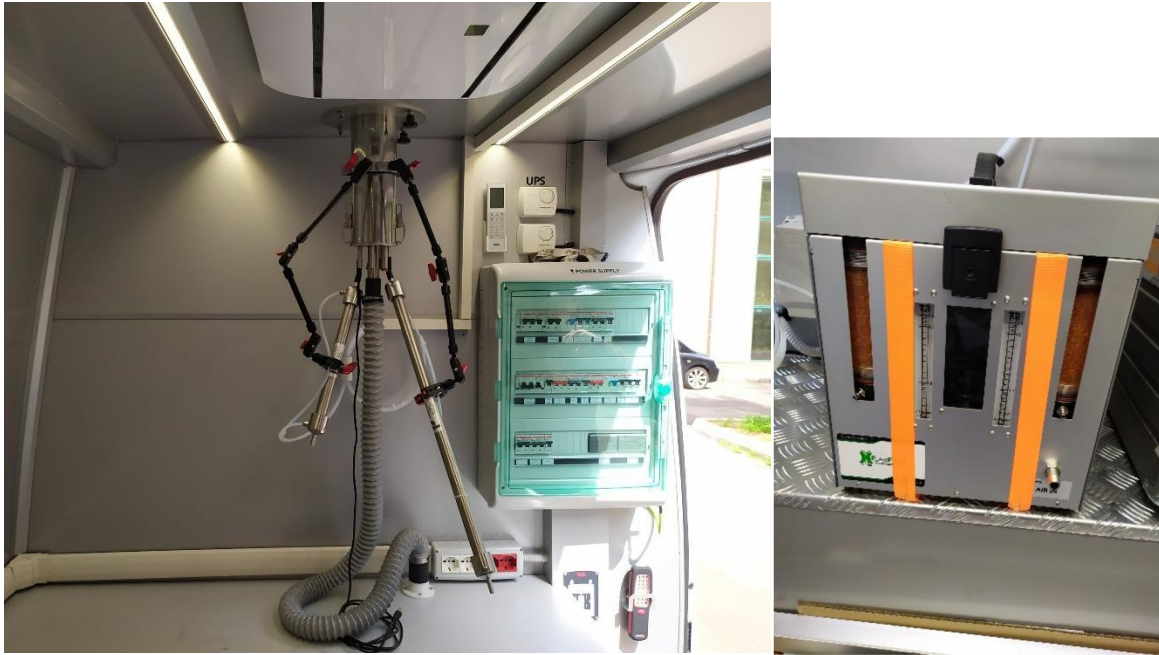
Figure 10: Pictures of the dehumidification system installed at the MAGA platform.
