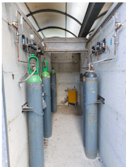
Figure 1: Gas cylinders (left: Air – right: Nitrogen) in the dedicated box.
