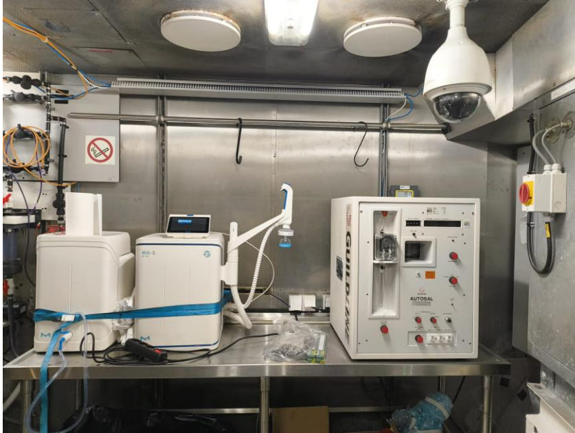
Figure 7. Installation of the salinometer in the Science Store on deck 1 of the R/V Gaia Blu.
