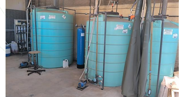
Artificial water production system
